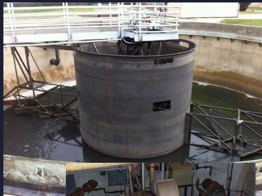
Primary equipment deteriorating
