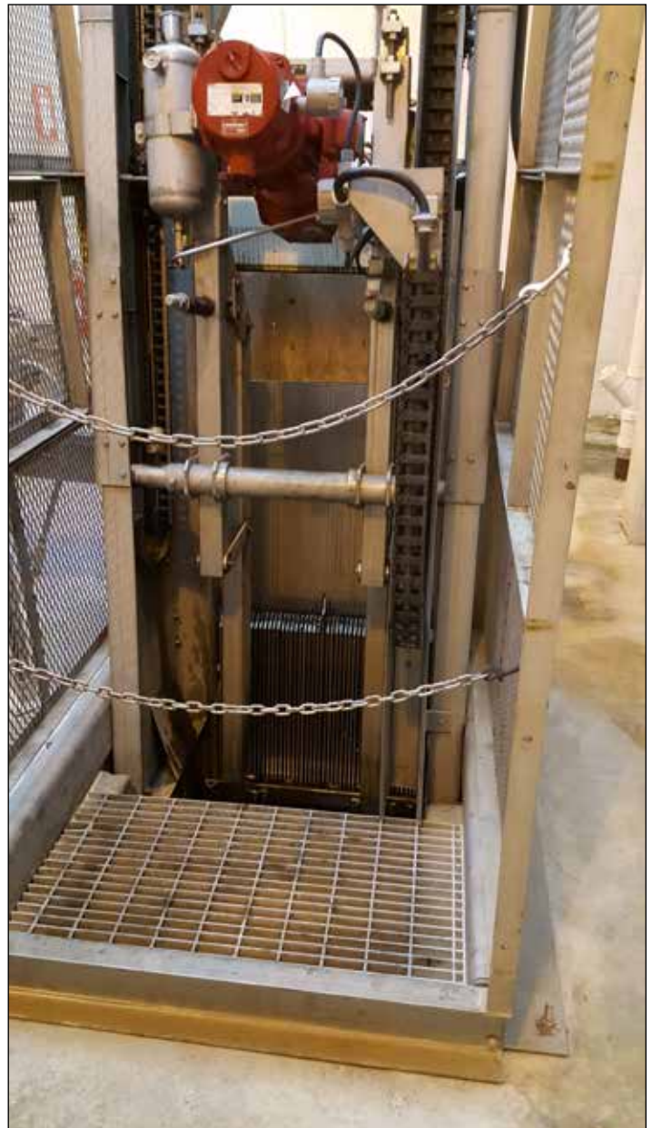
Influent Mechanical Screen
