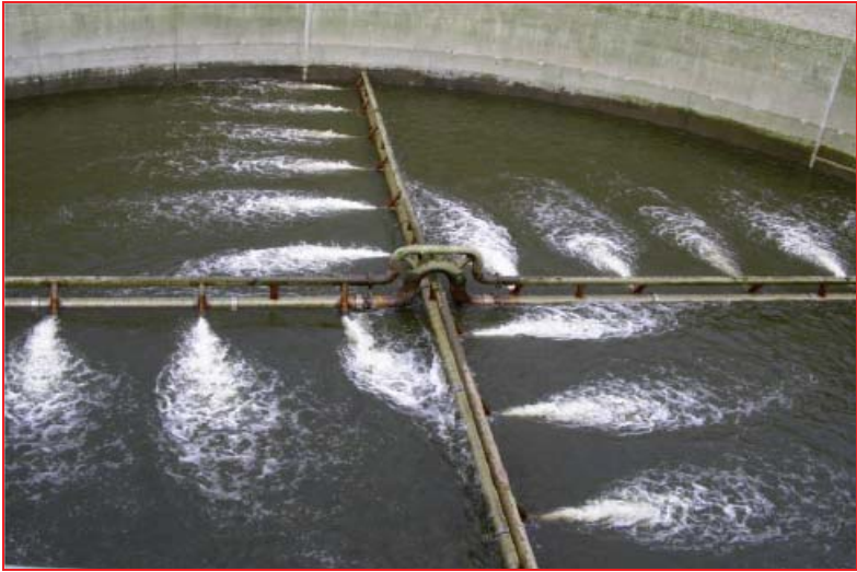
JET MIXING IN EQUALIZATION TANKS
