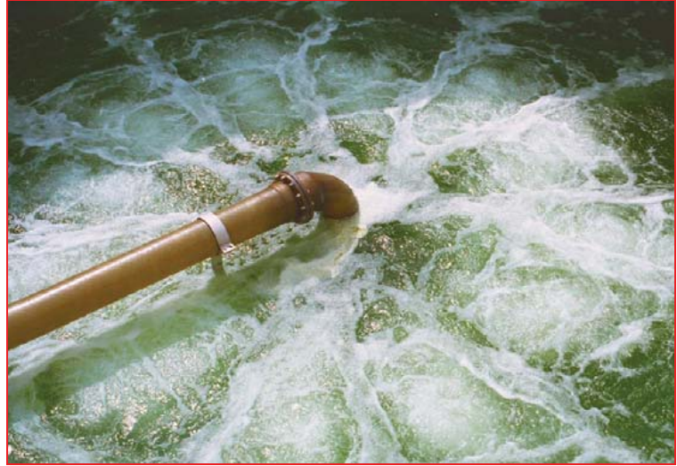
MIXING AND AERATION IN pH CONTROL TANK
