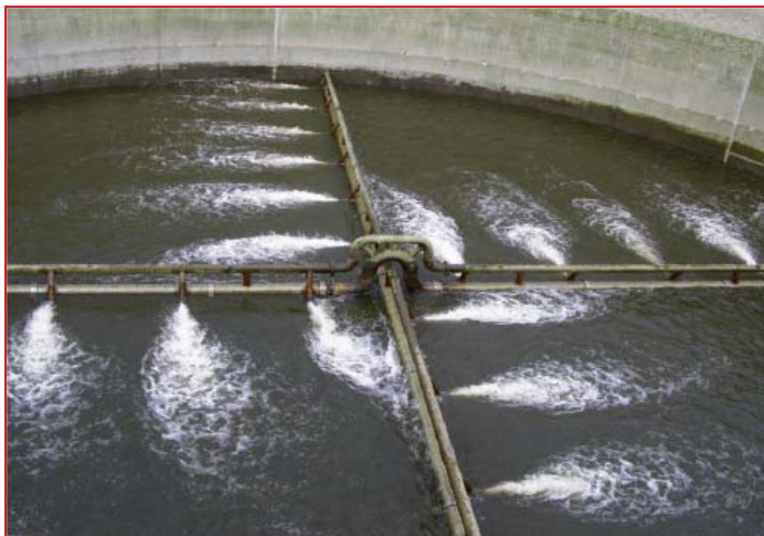
JET MIXING IN EQUALIZATION TANKS
