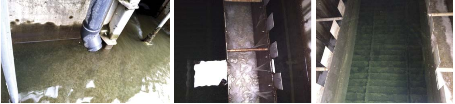
Figure 2: These pictures are of the high rate treatment system's influent (left) and effluent (middle and right) when adjustments were made after discovering the coagulant pumps were under-dosing with the help of the AF7000 Streaming Current Meter.
