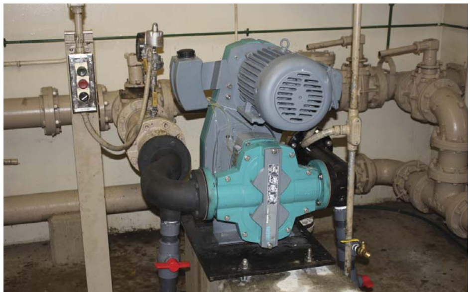
NETZSCH T2 Rotary Lobe pump installed in 2013 for sludge transfer from primary tanks to digester
