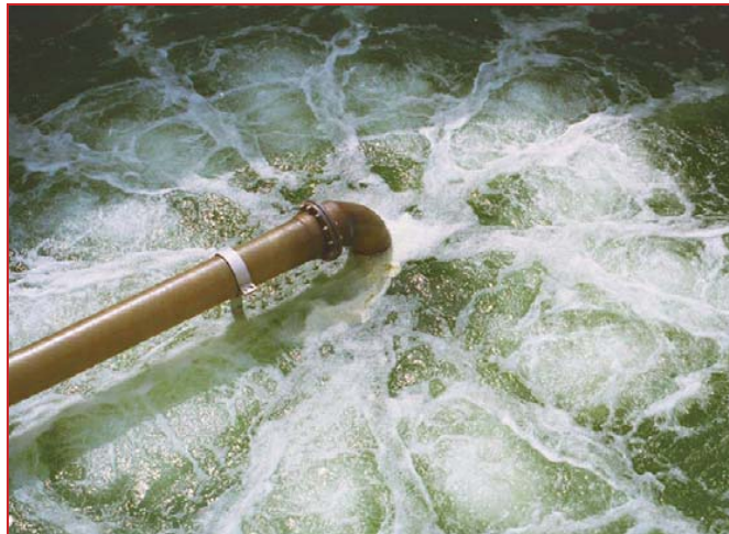
MIXING AND AERATION IN pH CONTROL TANK
