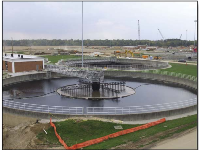
Secondary Clarifiers Southerly Wastewater Treatment Plant – Columbus, Ohio
